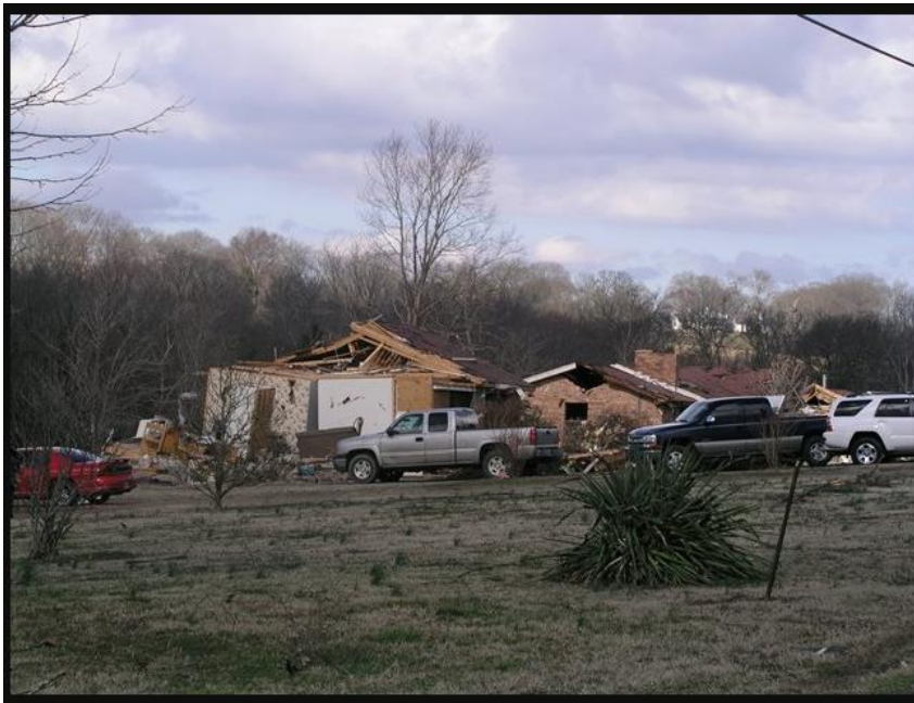
Figure 24: February 5, 2008 Tornado Damage residential homes (Source: The Tennessean)
